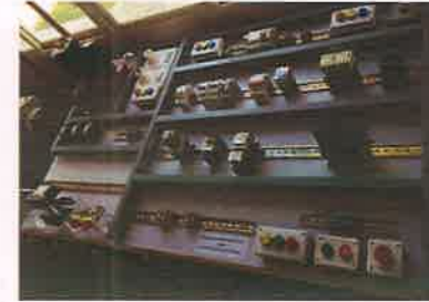
Specialized Training Equipment for Control Panel Wiring Training (In-house designed and developed) Installed at DDU-KK (Knowledge Dissemination)
